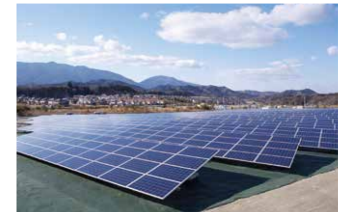
Kintetsu Hana-yoshino Photovoltaic Power Plant (Yoshino County, Nara Prefecture)
